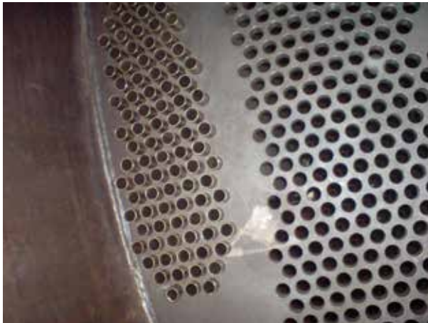
Fig. 7.15. Tubes of turbine's condenser (Source: WEB-7)
