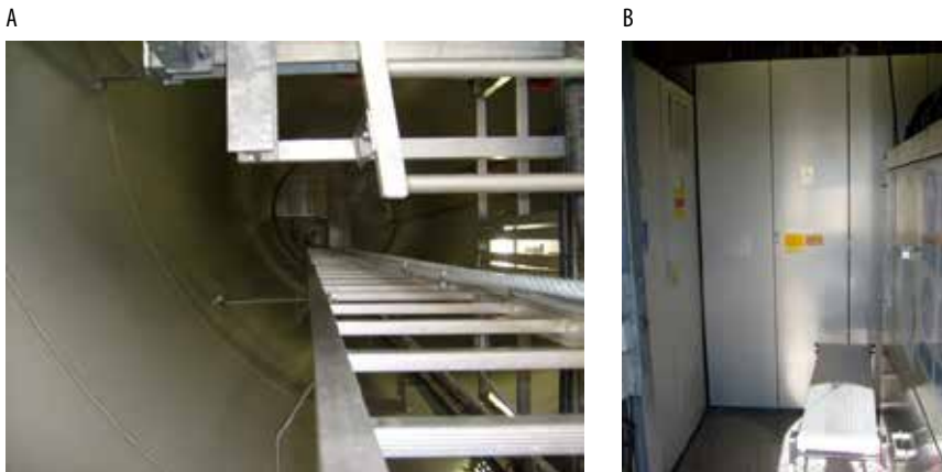
Fig. 3.19. The interior of a tubular steel tower A) service ladder, B) control cabinet (Source: photos by T.J. Teleszewski)
