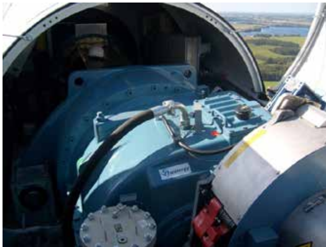
Fig. 3.20. View of the gearbox in a wind turbine gondola (Source: photo by T.J. Teleszewski)
