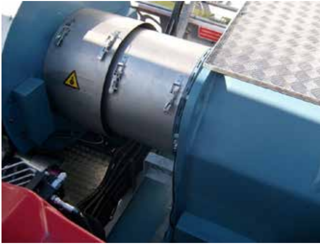
Fig. 3.21. A wind turbine coupling (Source: photo by T.J. Teleszewski)
