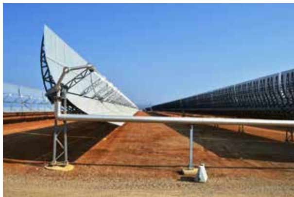
Fig. 2.33. Parabolic trough reflector plant "LA AFRICANA" in Cordoba (Source: photo by A. Rodero)
