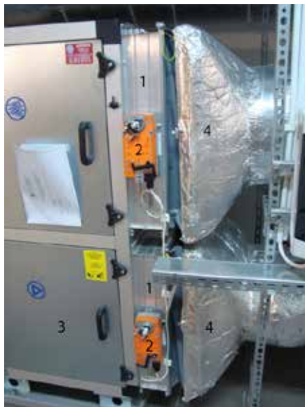
Fig. 8.13. An example of application of a throttle regulation: 1 – an air damper, 2 – an electric actuator, 3 – a fan, 4 – a ventilation duct (Source: T.J. Teleszewski's private archive)
