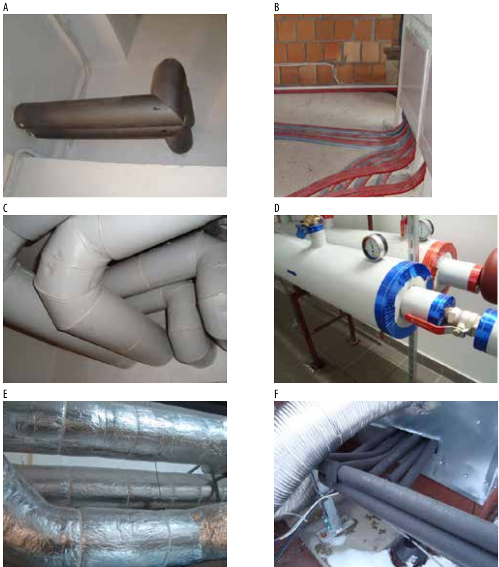
Fig. 7.17. Examples of insulation: A) foamed polyethylene without an outer coating, B) foamed polyethylene with an outer coating of polyethylene film, C-D) foamed polyurethane in a PVC housing, E) mineral wool with an aluminium foil coating, F) elastomer insulations (Source: A-CT.J. Teleszewski's private archive, D-E R. Bilinskiene's private archive)
