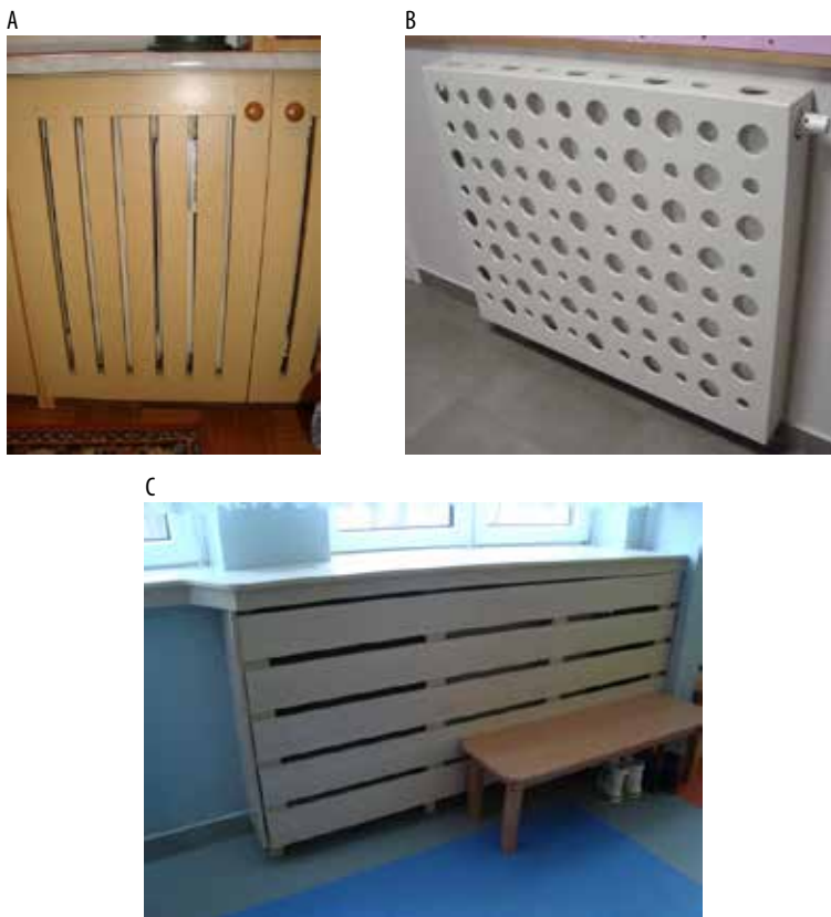
Fig. 7.10. Examples of radiator covers (Source: T.J. Teleszewski's private archive)
