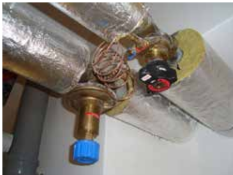
Fig. 7.15. An example of a direct-operated pressure regulator installed on a central heating system (Source: T.J.Teleszewski's private archive)
