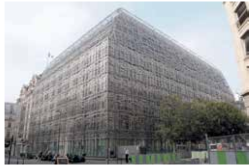
Fig. 1.29. Surrounded by a stylized metal structure, the building of the French Ministry of Culture (Paris, France) (Source: photos by M. Kłopotowski)
