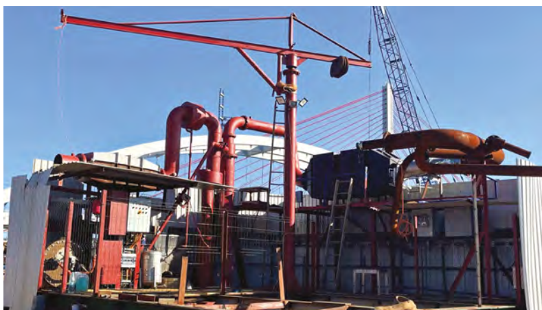
FIGURE 10. Photograph of the tested flue gases cleaning system fitted with multi-jet scrubber
