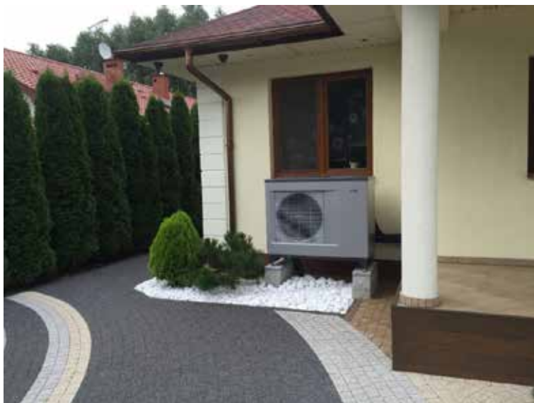
Fig. 5.29. An example of the air heat pump – external unit (Source: Smuczyńska, 2015)
